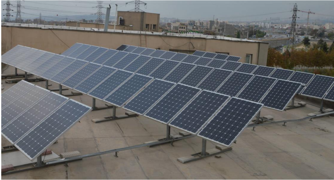
Fig. 3. Photovoltaic panels of the Abbaspour School of Engineering.
